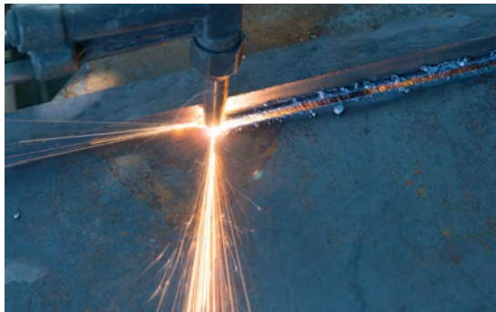
Hot surfaces during metal cutting
